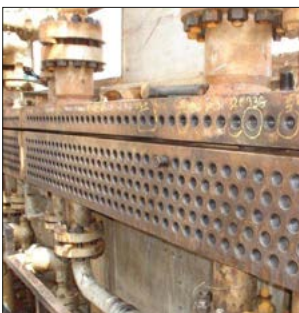
FinFan cooler before a maintenance
